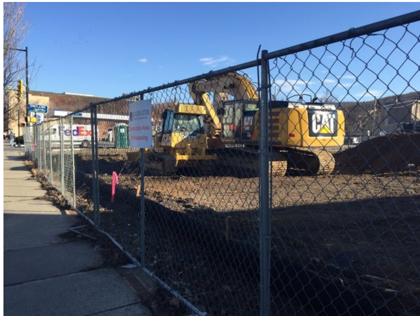
Construction is already underway at the corner of Third and New streets in South Bethlehem.(Sara K. Satullo | For lehighvalleylive.com)
